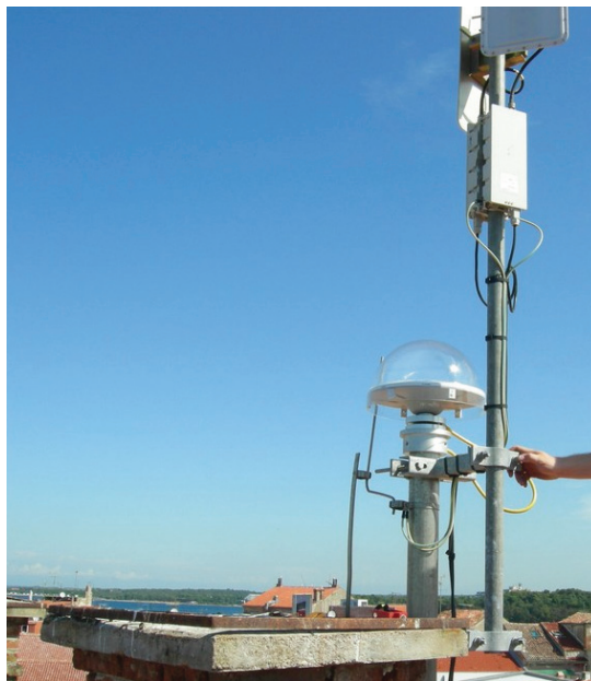
Figure 5. GPS aerial instalment for Poreč reference station
